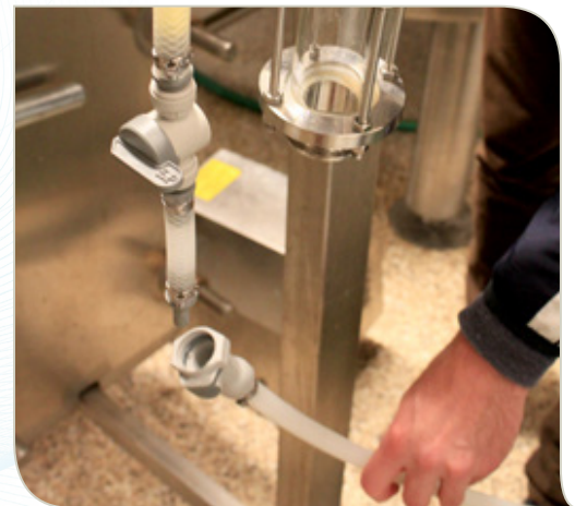
Quick disconnects from CPC are used to connect fluid and air lines in the brewing process at Urban Growler Brewing Co.
